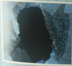
Windows break at level 5
